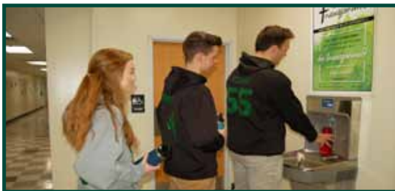
A new Elkay water bottle filling station was installed on the second floor in January for use by Upper School students and staff, a gift from ACS parents Dr. Salaam and Lauren Alobeidy and plumbing services donated by ACS parent Phil Kates.
